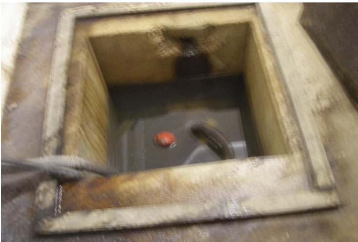
Sump pump in the cellar floor, half full of water.
