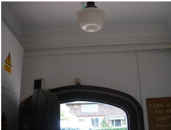
Damp around the front door in the porch area.
