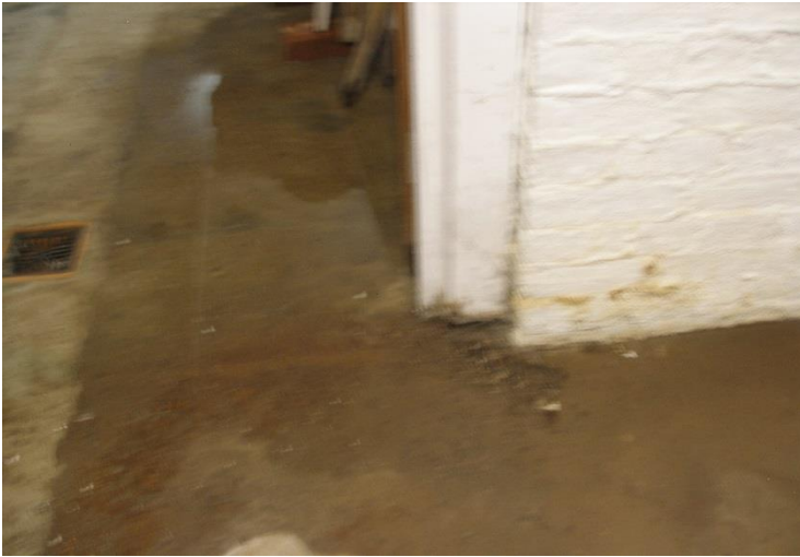
Surface water and gully in the cellar.
